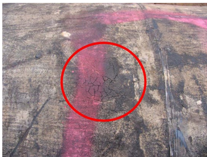
Figure 2. Cracks in the coating due to aged bitumen.
